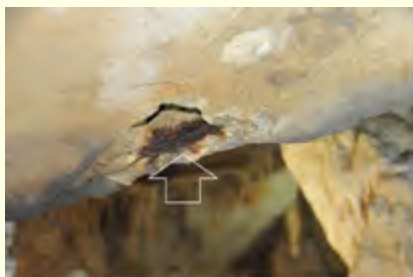
Photo of an area below a trail where the iron has rusted, resulting in damage to the concrete.
