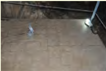
Many lamps would be replaced to a better positions, as this one installed on the floor of the passage, as well as their colour temperature should be standardized as white light (preferably 4000 K).
